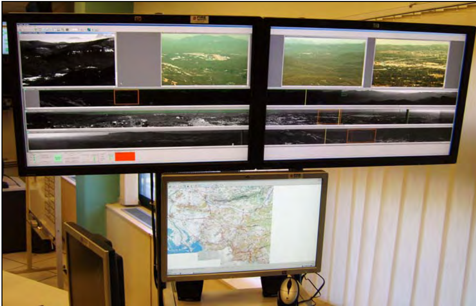
Automated rapid fire detection control panel of the “Fire Watch” system at SDIS13
